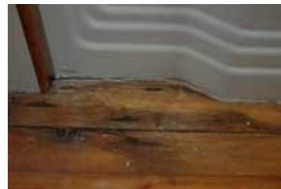
Water splashed outside a tub enclosure causes a common mold environment, indicated by black staining on the floorboards. Noelle Lord photo.
