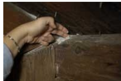
Thanks to roof leaks and faulty gutters, a healthy deposit of mildew is thriving at this attic-timber intersection. Noelle Lord photo.
